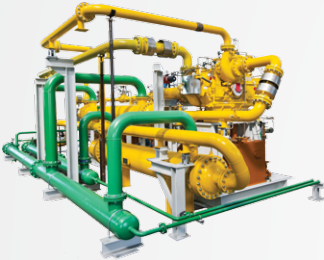
The three-stage MSG-3 compressor pictured above boosts the pressure of natural gas entering power generation turbines at a combined cycle power plant in Russia
